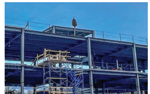
Bonnette, Page & Stone team members position a tree on top of the steel structure at 51 Elm Street, Owner Paugus Properties' future mixed-use building located in Lakeport, NH.
